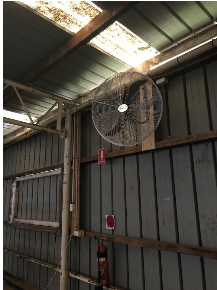
Fans in the Peden Pavilion
